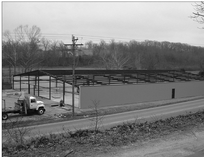
The metal structure for the new Barry County Museum stands out against the winter landscape on Highway 112 south of Cassville.
